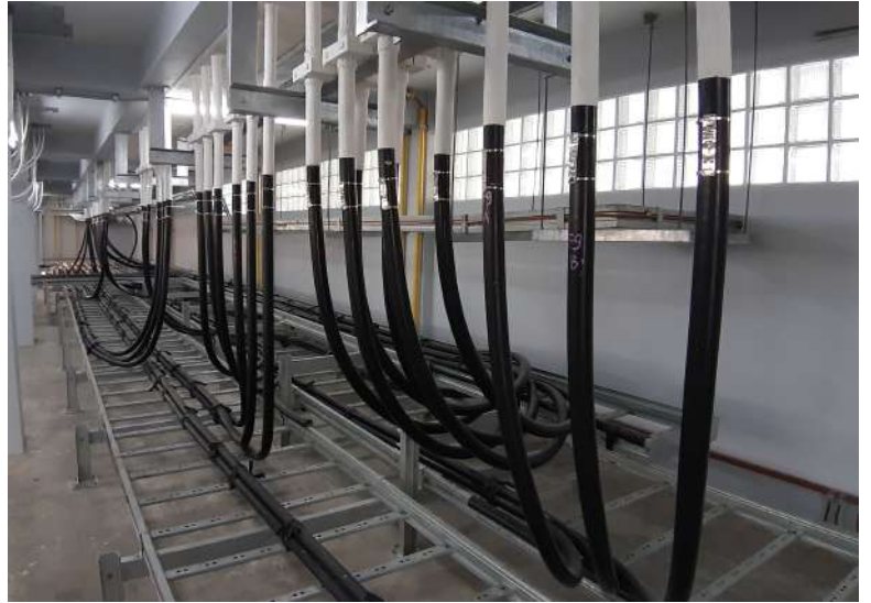
“H.V. POWER CABLE 22 kV SUBSTATION”
